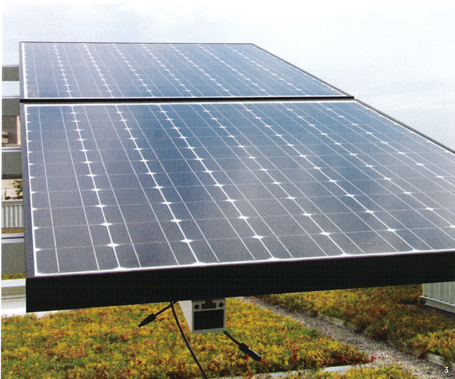
PHOTOVOLTAIC ARRAYS ARE MOUNTED ON THE GREEN ROOF. TOGETHER WITH A WIND TURBINE, THEY PROVIDE ABOUT 7KW OF ELECTRICITY [3].
